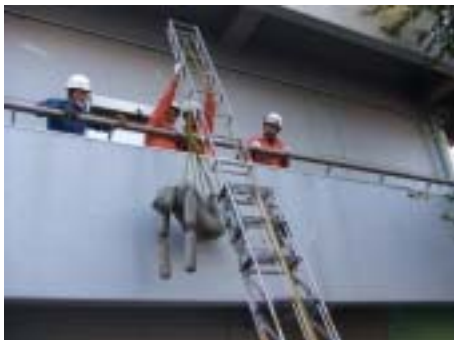
Photo7: Emergency Ladder Rescue
